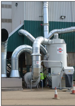
Wet scrubber VDN-AS with de-sludging de
